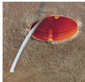
The KBT... box with terminated conductor ready for mounting the KBP... chandelier hook.
